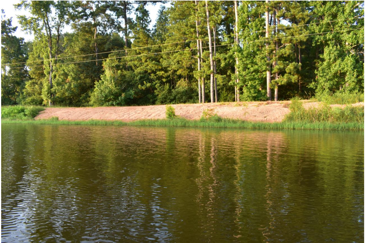
Figure 12 - Low area close to the spillway Before erosion control mat
