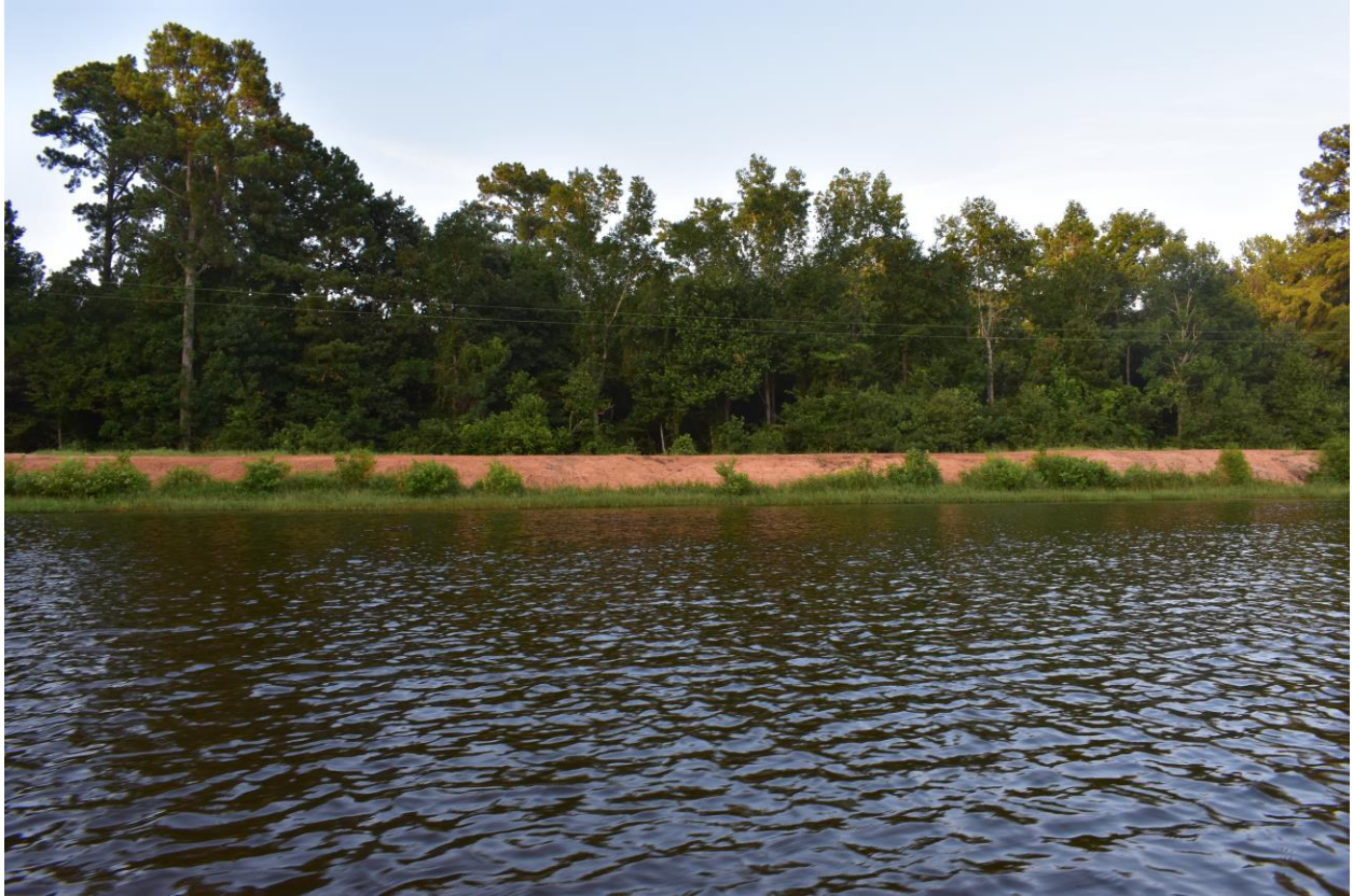
Figure 17 - Front of the low flow pipe and hog damage. Before erosion control mat
