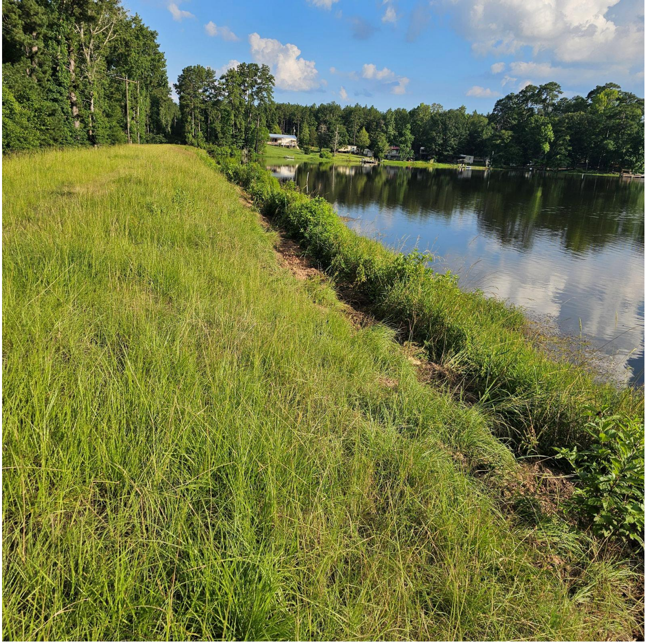
Figure 11 - Hog damage. Before work was done
