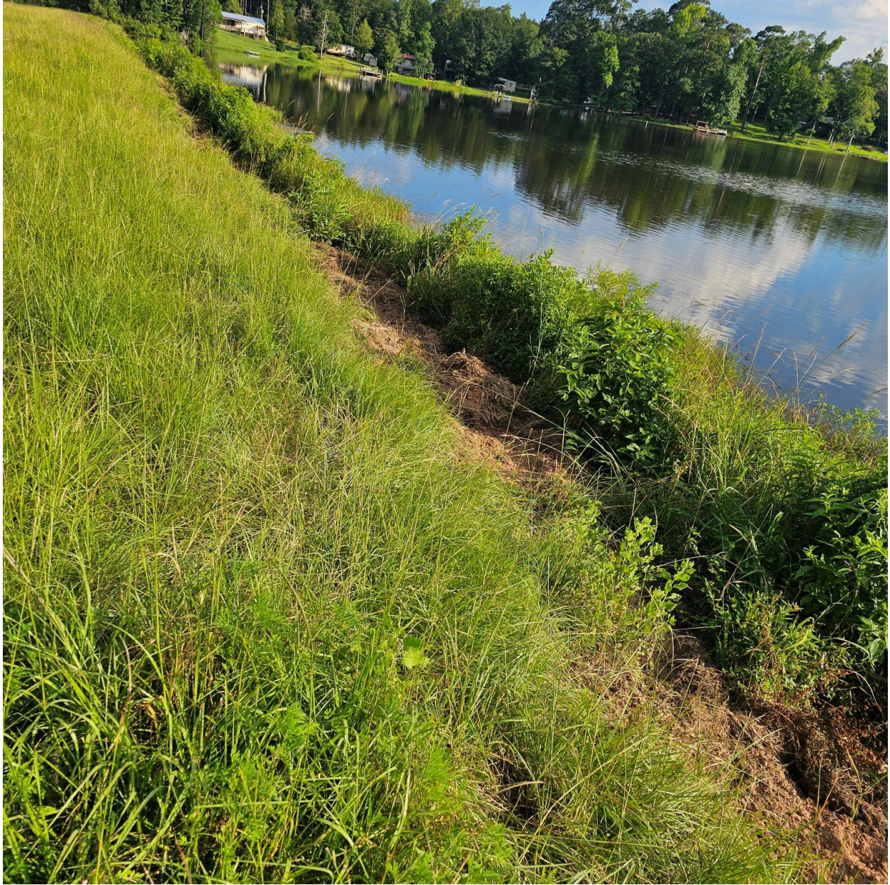
Figure 10 - Hog damage. Before work was done
