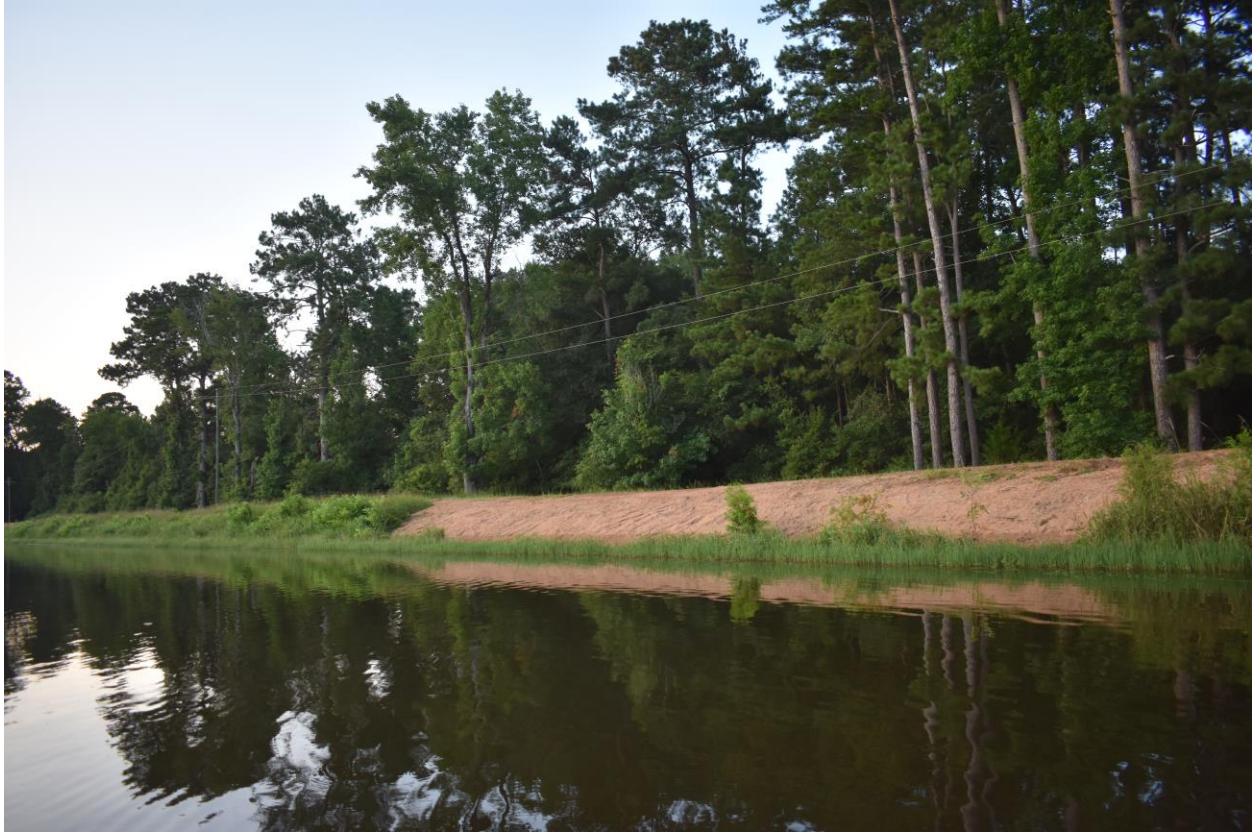
Figure 13 - Low area close to the spillway Before erosion control mat
