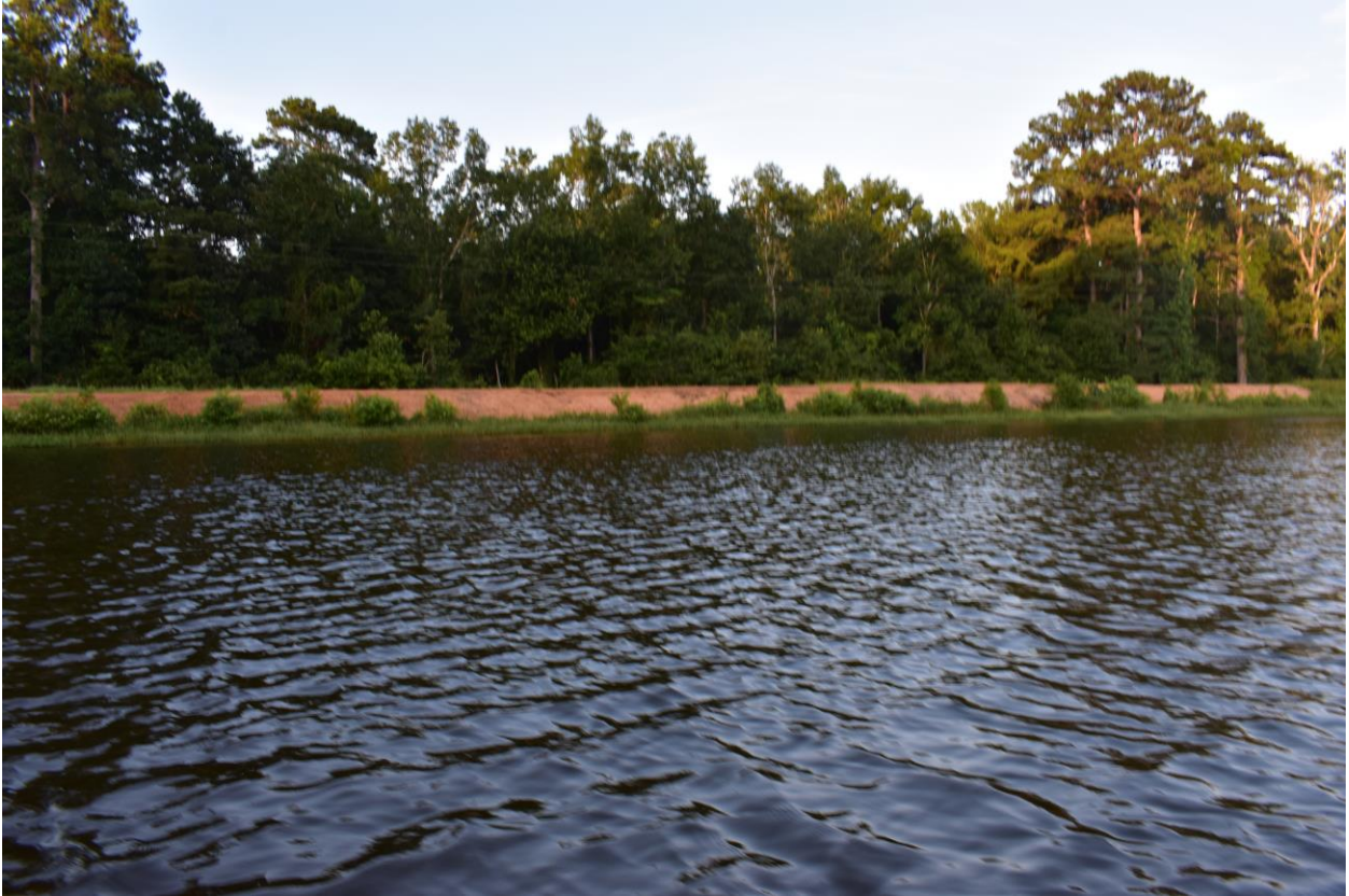
Figure 16 - Front of the low flow pipe and hog damage. Before erosion control mat
