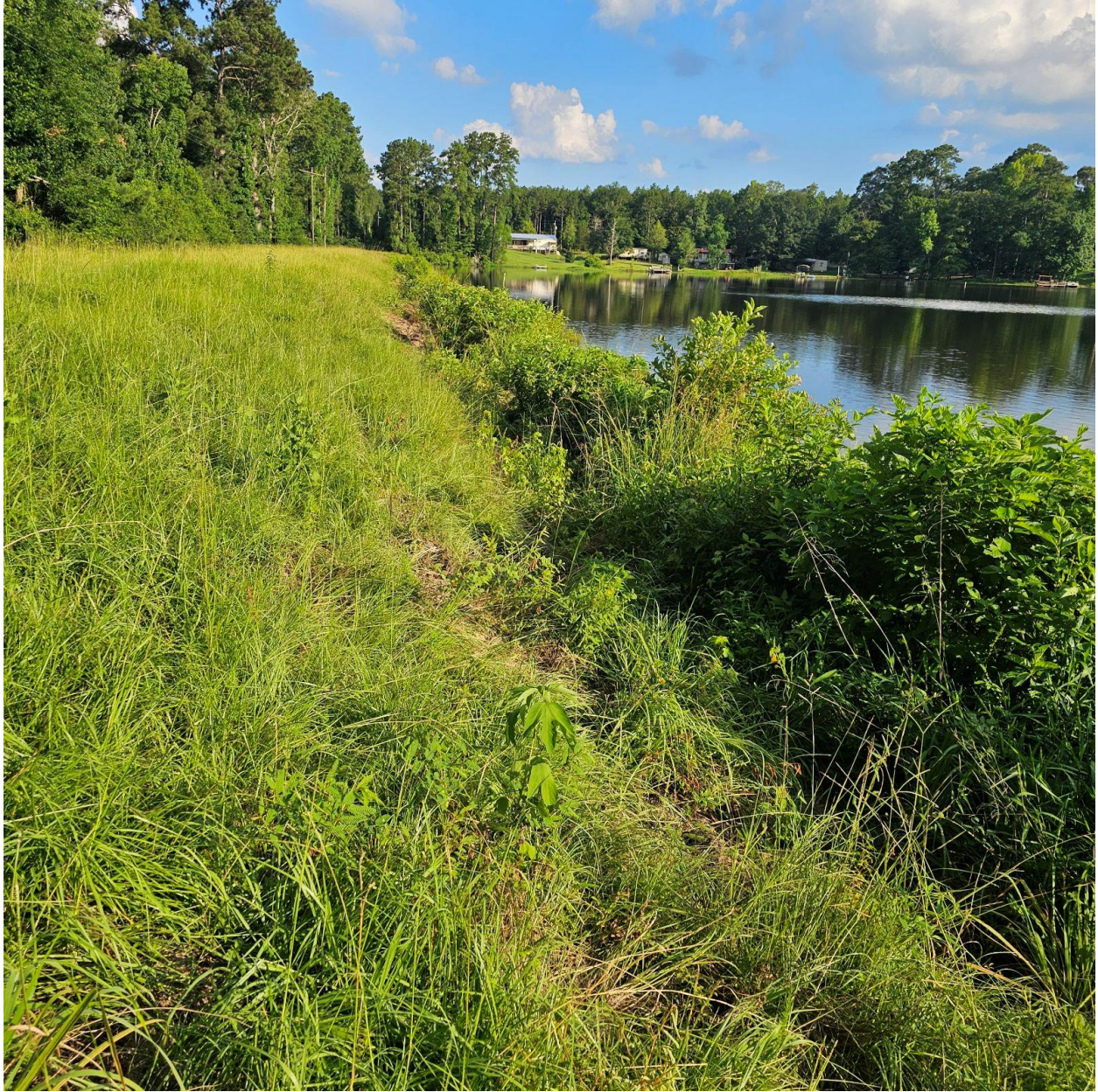
Figure 7 - Hog damage facing South. Before work was done
