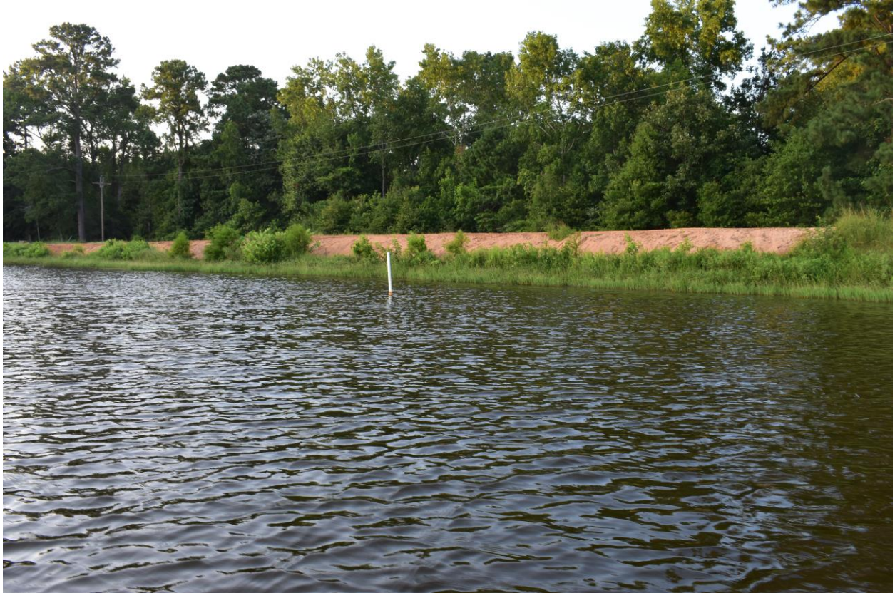
Figure 15 - Front of the low flow pipe and hog damage. Before erosion control mat
