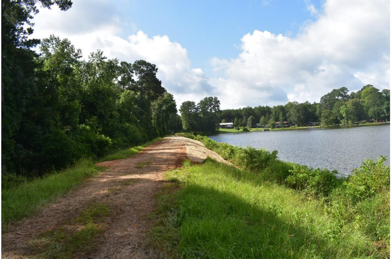
Figure 25 – Top side where hog damage occurred. After the erosion control mat
