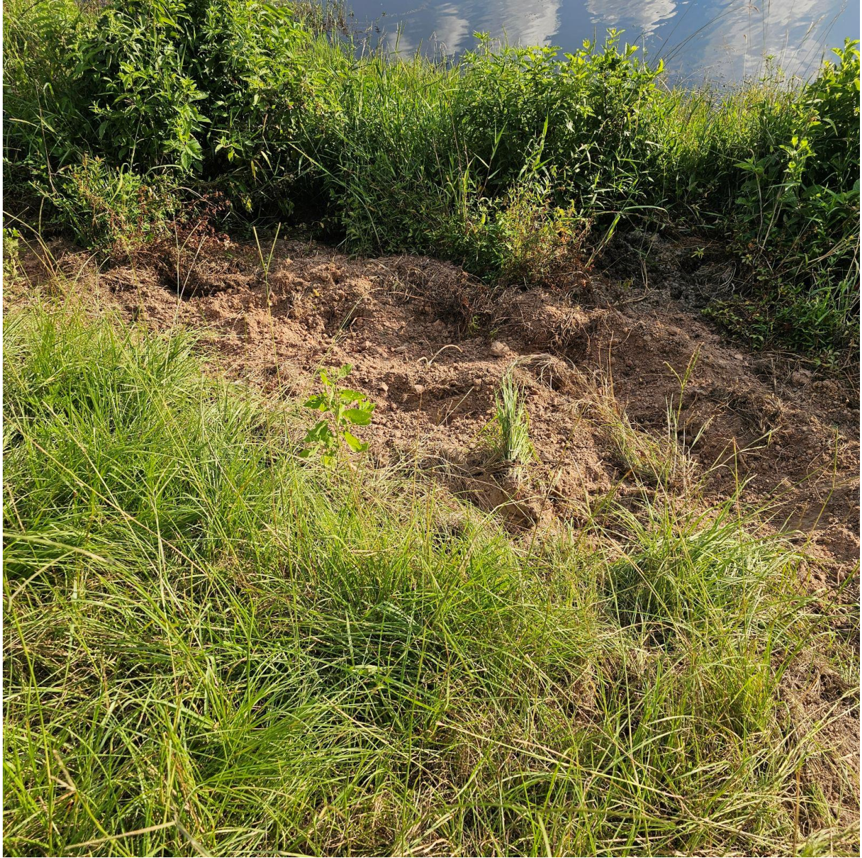
Figure 9 - Hog damage. Before work was done
