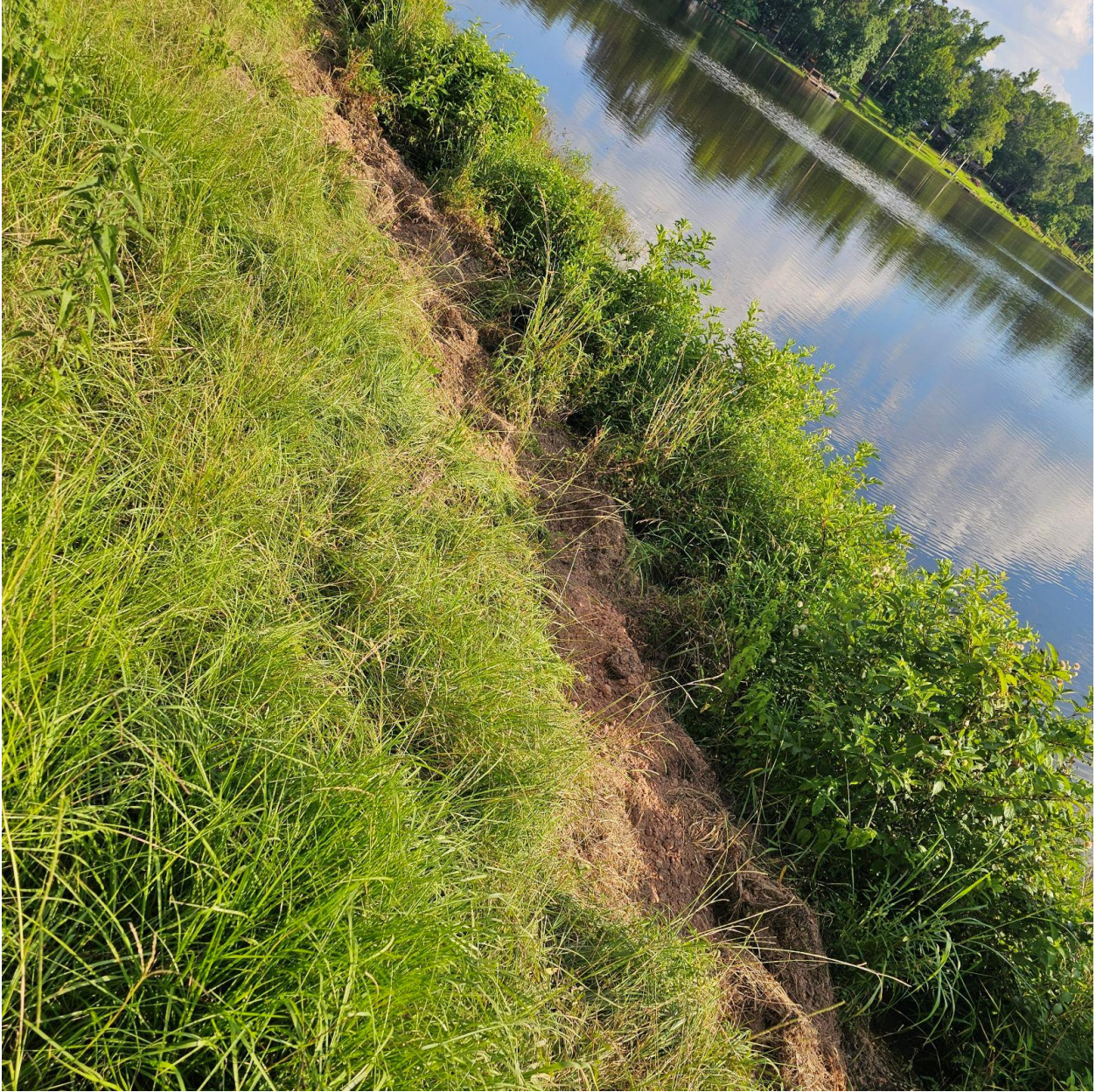
Figure 8 - Hog damage facing South. Before work was done
